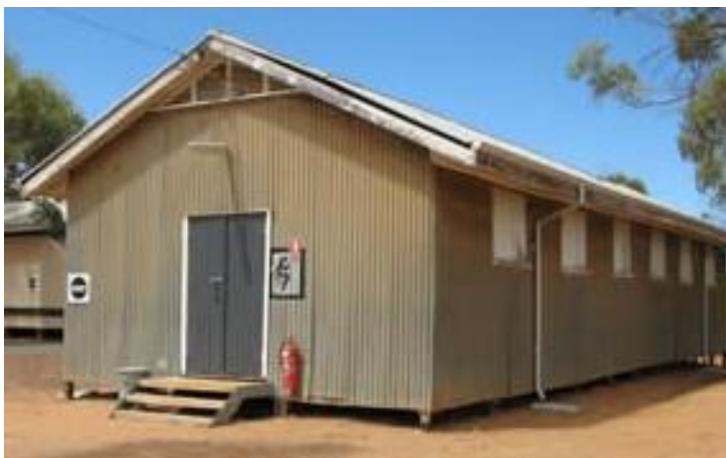
A standard configuration P1 hut still in use at Northam Army Camp in 1980
